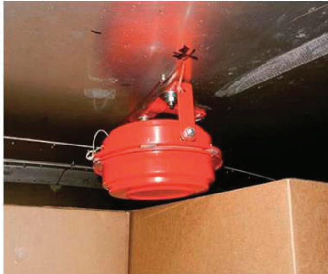
Figure 6.2. In-container fire suppression system
